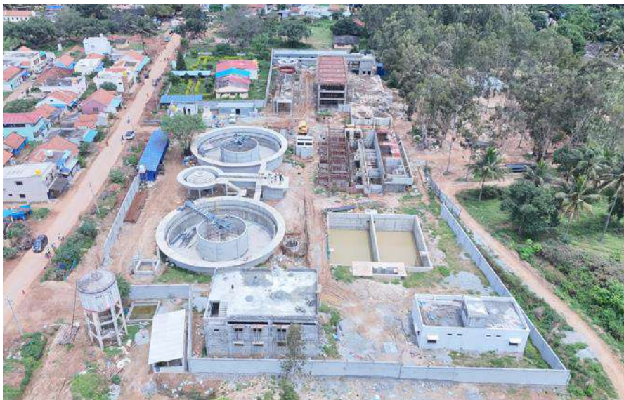
17.70 MLD WTP at Hassan, Karnataka
