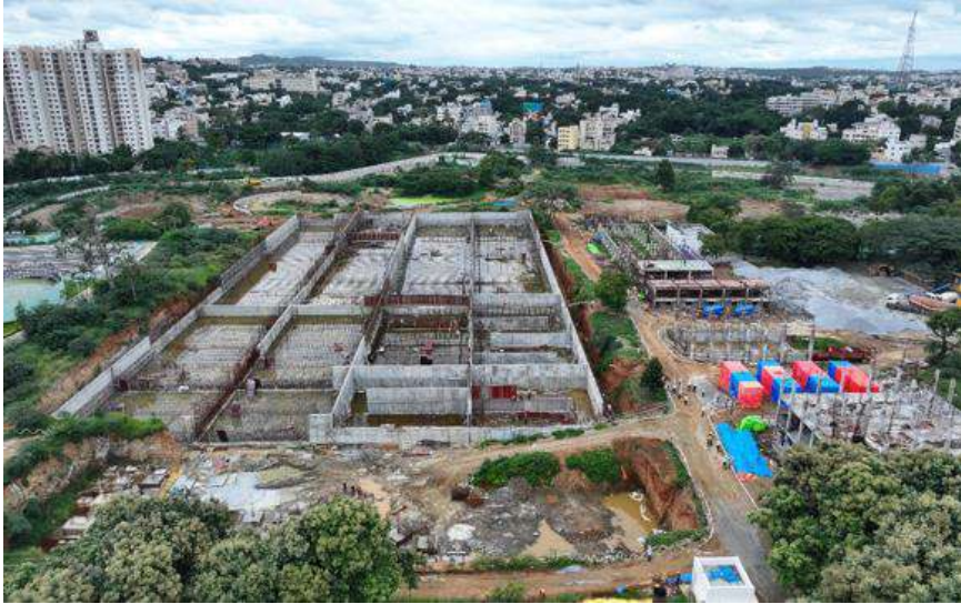
150.00 MLD STP at V Valley, Bengaluru
